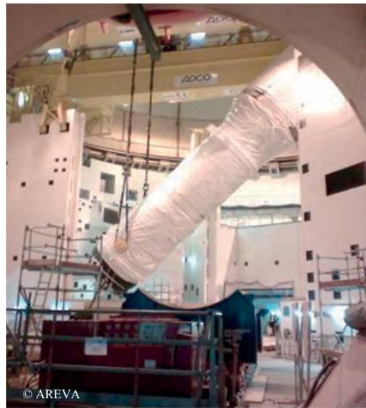
Fig. 5: Introduction of the second Steam Generator into the Reactor Building at Flamanville 3 EPR reactor, France.
